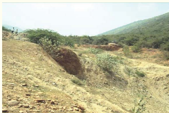
Eastern Main Canal at Km 6.00 to 10.00 delayed due to non acquisition of Forest Land
