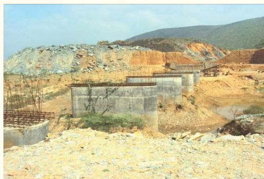
Non completion of CM & CD 21 works (Aqueduct)
