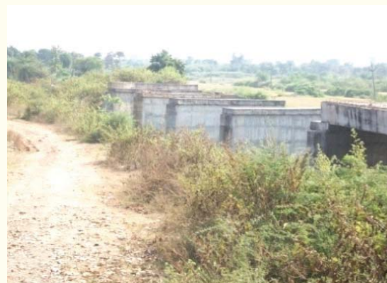
Incomplete bridge at Km 24.284 of FFC (Package-88)
