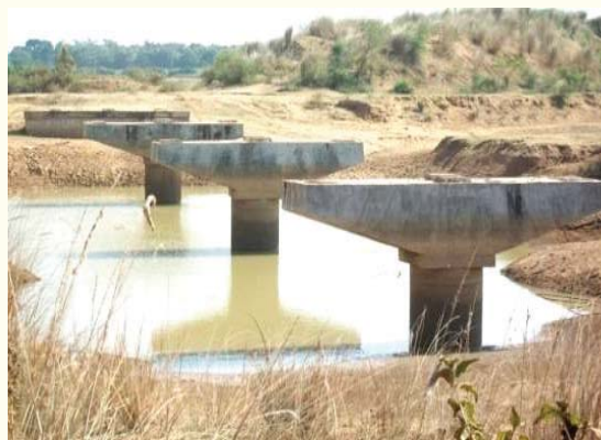
Incomplete bridge at Km 13.062 of FFC (Package-87)
